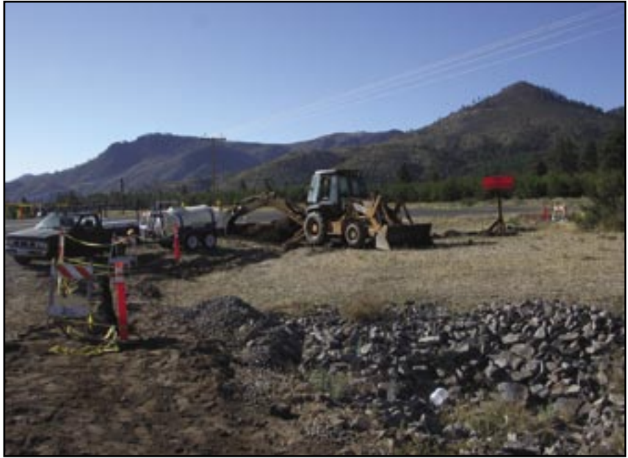
Figure 95—Rubber tire backhoes are an integral component of storm inspection and response.
